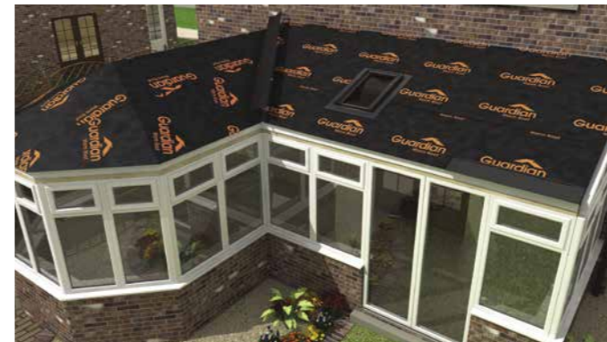
Breathable waterproof membrane is laid over the plywood and secured in place.
